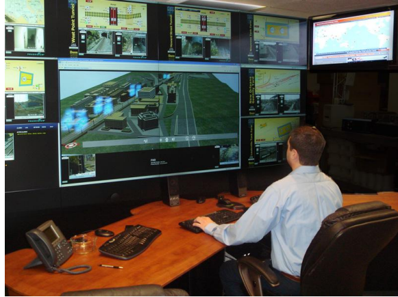
Command and Control Center
